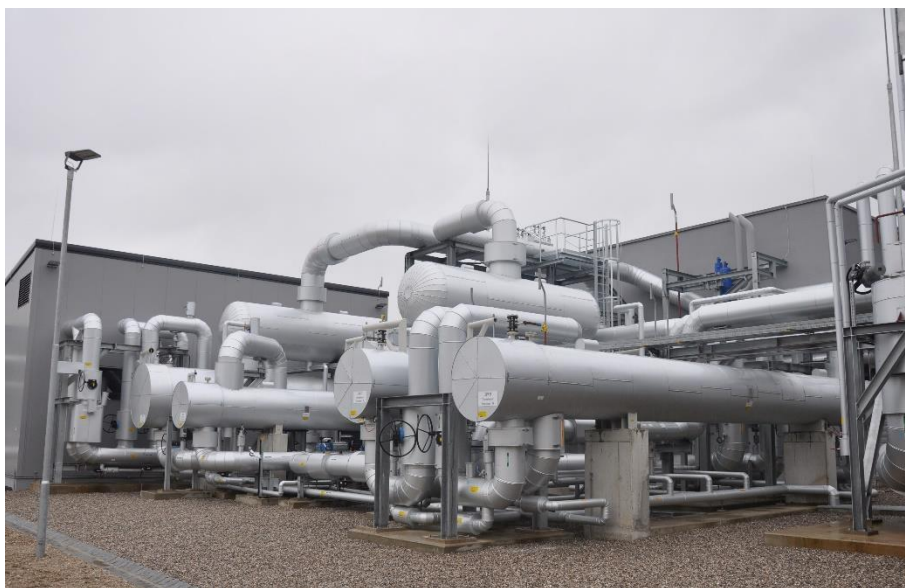
Geothermal power plant, Garching a.d. Alz, Germany – copyright Strabag
